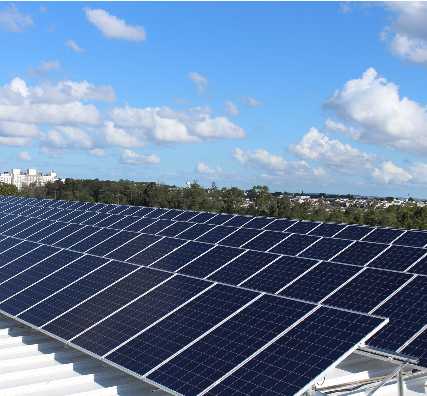
Solar panels at ParkShopping Canoas, in Rio Grande do Sul
